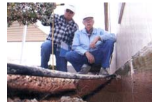
Leon Henager, left, and Clyde Preston stand near one of the sinkhole problems.
